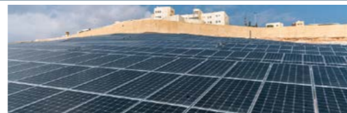
Energy efficient The new solar farm powering SESAME.
